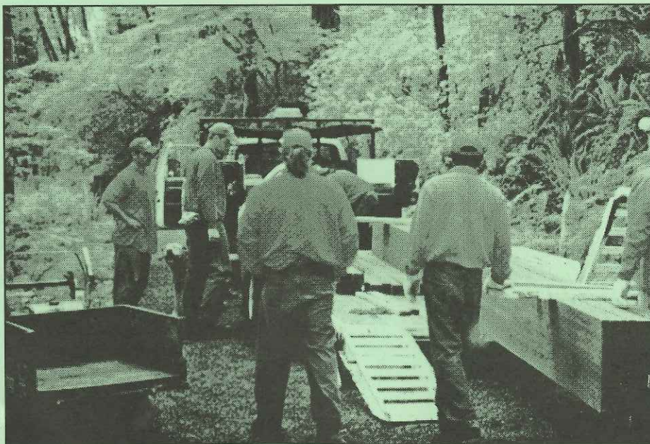
DNR crew moving 25-foot beams for bridge #1 on the Bells Mtn. Trail
